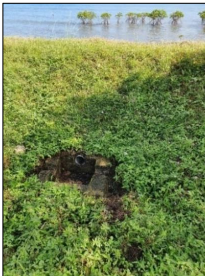
Figure 4.5 The drainage point behind the Vusasivo Village seawall often becomes overgrown and blocked with leaves which contributes to flooding in the village (Source: Author, 2022).
