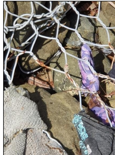
Figure 4.6 Broken and rusting wire in the seawall built in 2015 at Vusasivo Village can be a potential health risk to community members, no longer holds the rocks in place, and causes waste to become trapped (Source: Author, 2022).
