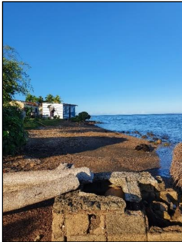
Figure 7.4 Several houses in Naivaka have been damaged by coastal erosion and inundation including this home in the foreground where the kitchen is located below the now high tide mark (Source: Author, 2022).
