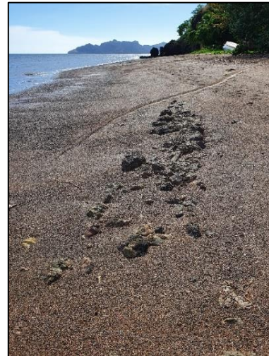
Figure 7.5 Remnants of the foundations of a never-completed seawall on the foreshore of Naivaka that was built during the 1980s (Source: Author, 2022).
