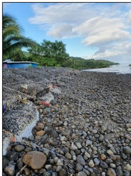
Figure 4.2 The seawall at Vusasivo that was completed in 2015 is made of small to medium-sized rocks held together by wire but has been damaged causing the rocks to fall away (Source: Author, 2022).
